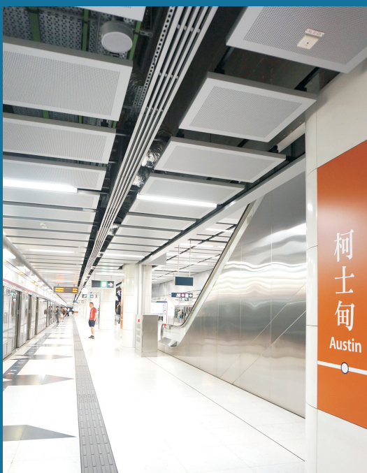
Austin MTR Station Ventilation System
